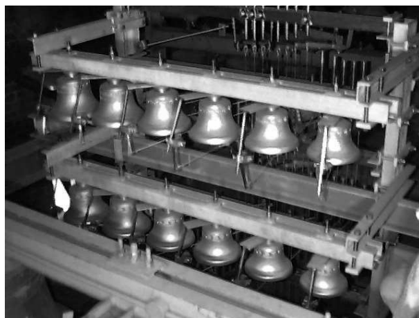
Fig. 3. The twelve, new installed carillon bells (control levers of mechanical action are visible).
